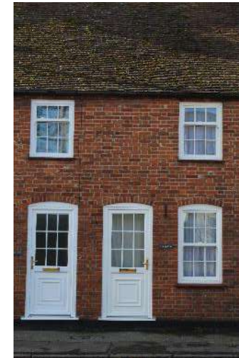
Figure 76 Loss of Architectural Details
